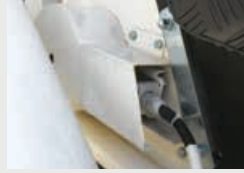
LIMIT SWITCH HOPPER GRID
