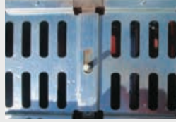
GRID PROTECTION WATER BOX
